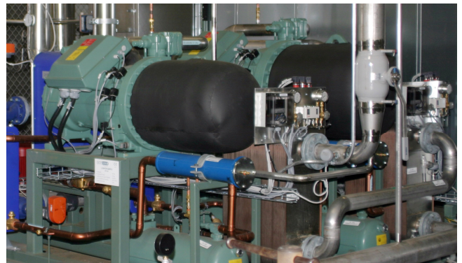
The HP-unit installed in Riihimäki.
